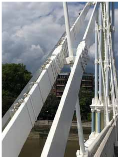
Bazelgette's vertical strengthening rods with the original Rowland Mason Ordish 1874 Albert Bridge design.
